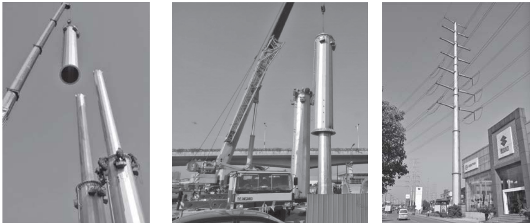
a) Lifting the outer tube; b) Placing the outer tube; c) Pole in service.
